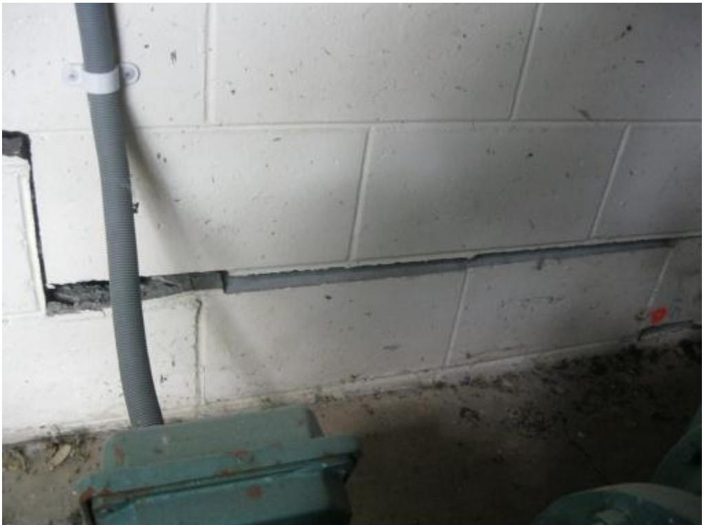
Photograph 6: Damage to external northeastern wall.
