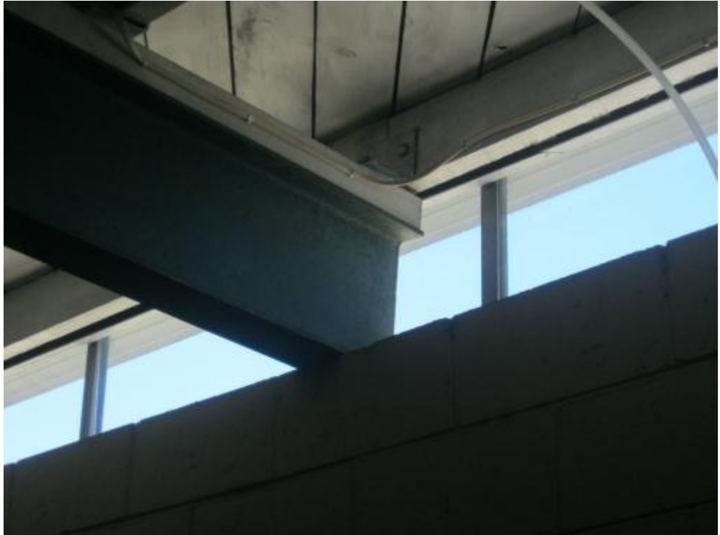
Photograph 13: Steel rafter rollover damage.
