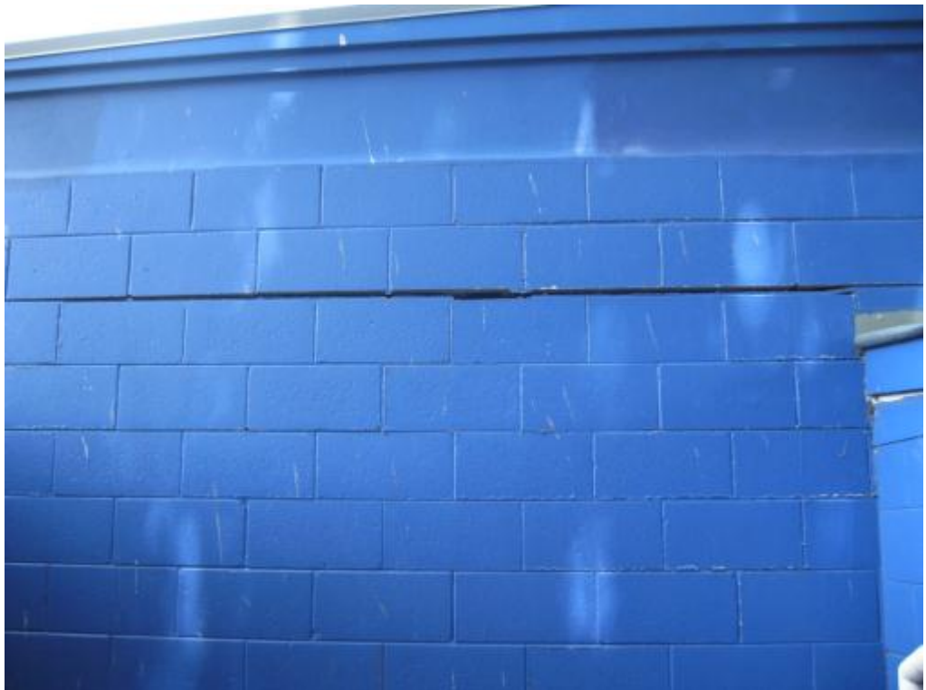
Photograph 8: Settlement damage at southern side of northeastern external wall.
