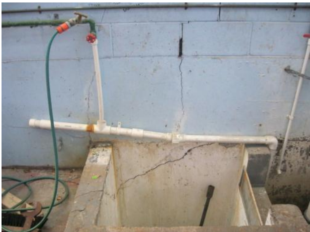
Photograph 12: Damage to wall and foundation at service pit.
