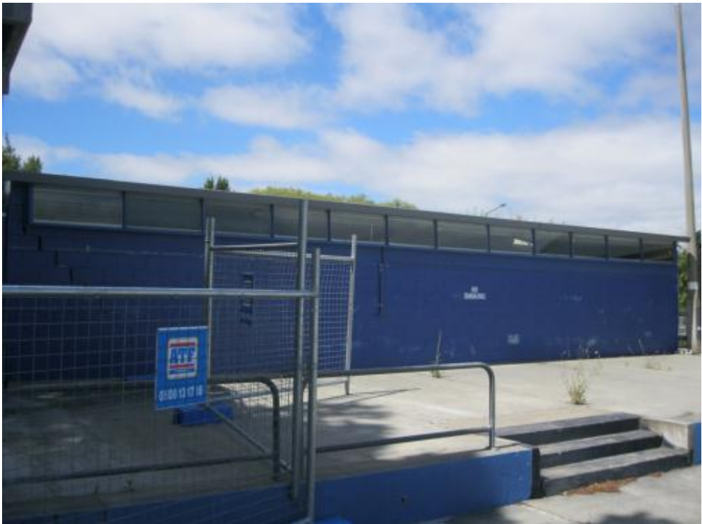
Photograph 2: Northwestern exterior wall elevation (damage at left).
