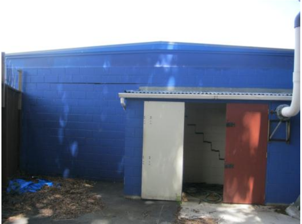
Photograph 3: Northeastern exterior wall and addition – note settlement and lateral movement.
