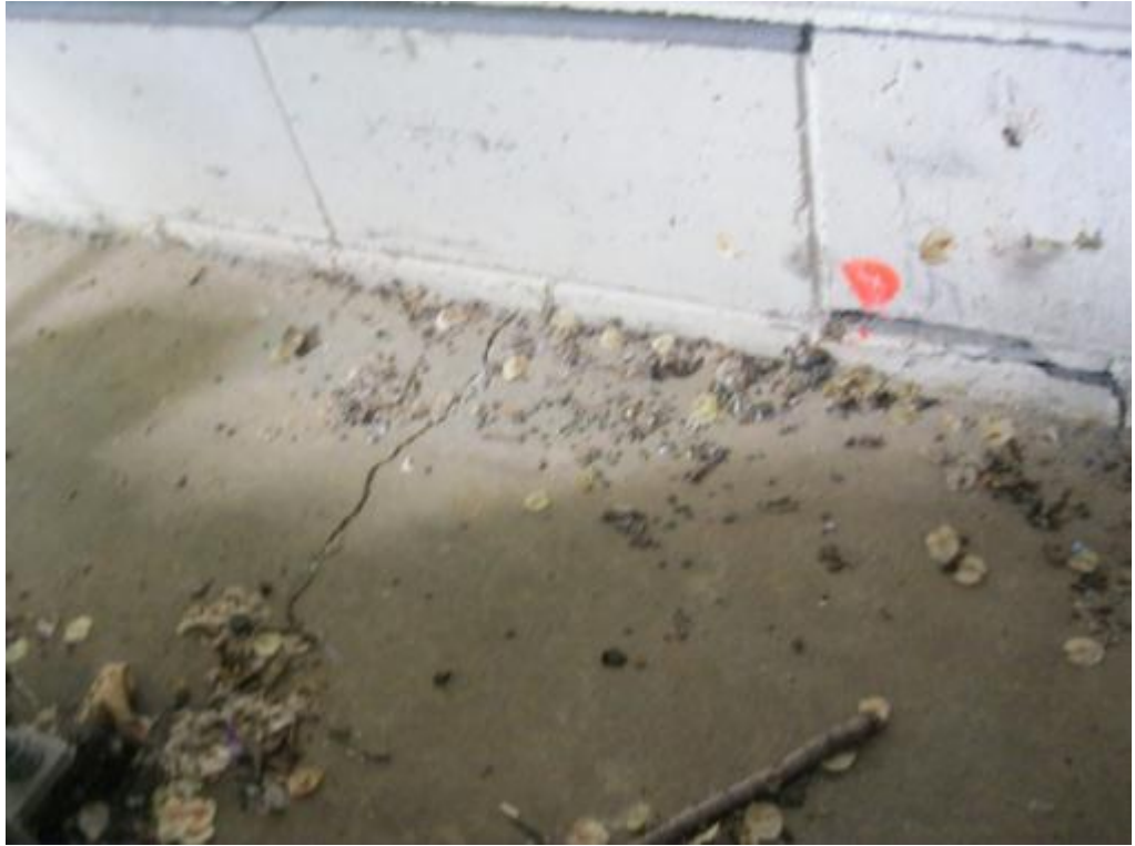
Photograph 7: Floor cracking at northeastern external wall.
