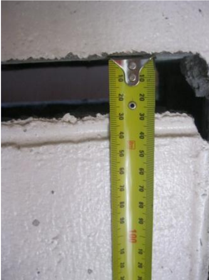
Photograph 5: Damage to northeastern exterior wall (inside addition).
