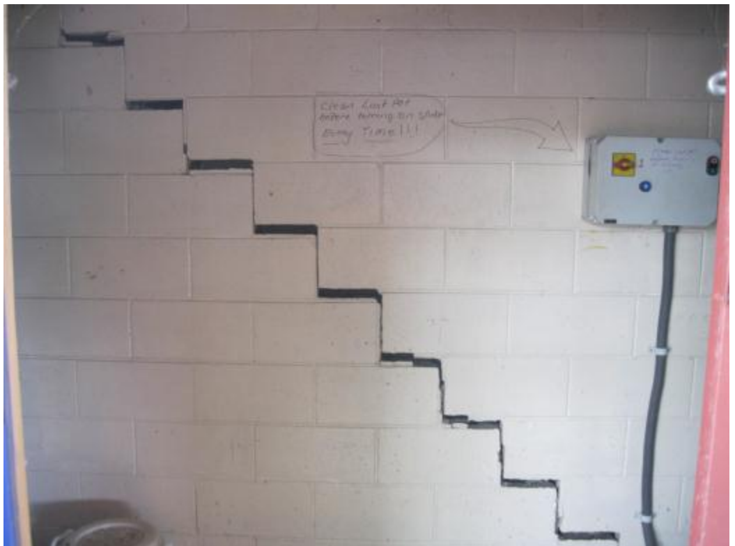
Photograph 4: External view of northeastern exterior wall damage (inside addition).
