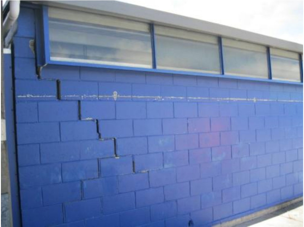
Photograph 1: Northwestern exterior wall shear damage.
