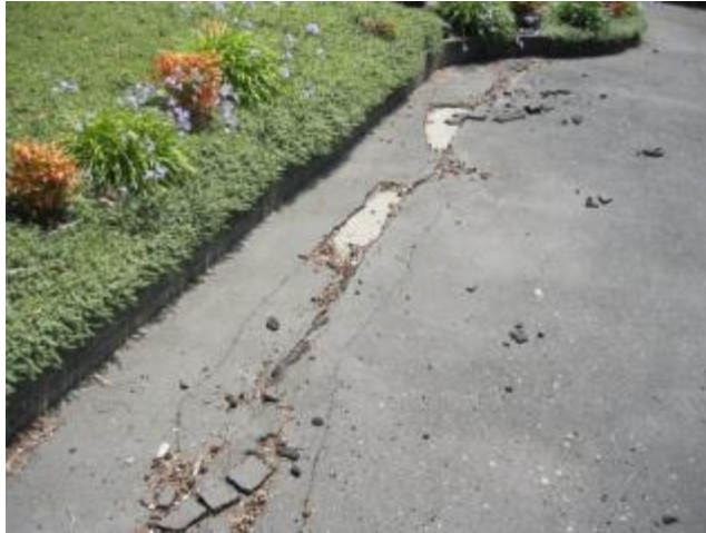
Photograph 7 Cracking in asphalt paving roadside, possible lateral spread.
