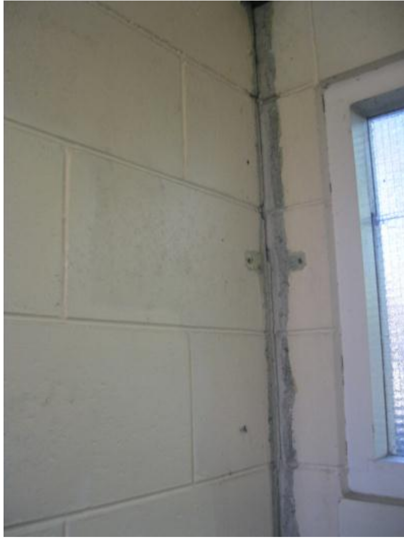
Photograph 7 Existing cracking at connection between a transverse wall and a longitudinal wall
