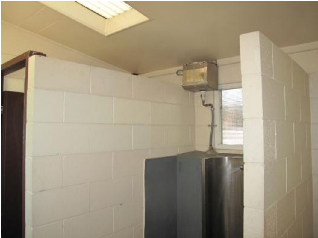
Photograph 5 Unrestrained partial height concrete masonry walls
