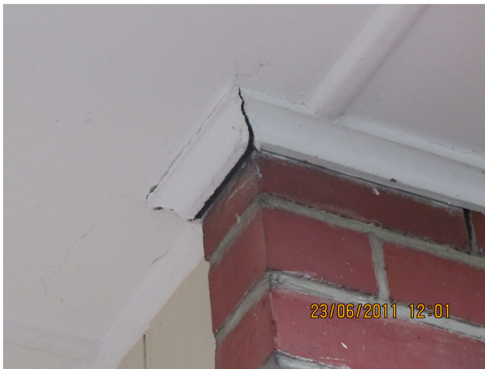
Photo 4 – Typical masonry veneer damage
