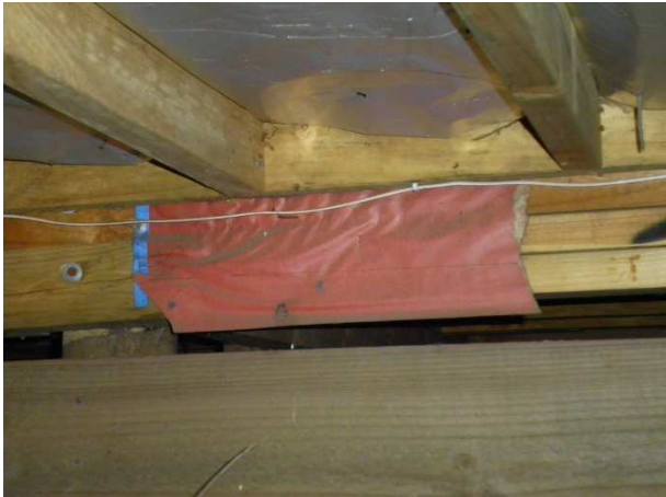
Sagging floor structure below office at south end.
