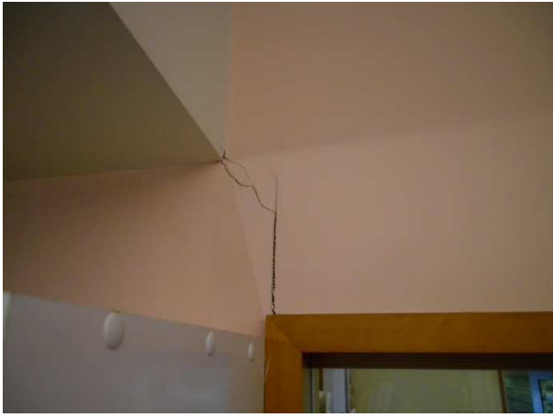
Crack adjacent to door opening in office.
