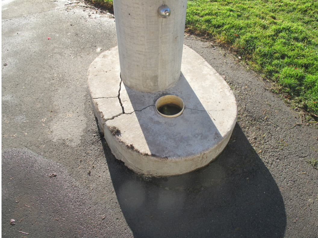
Photograph 5 Cracking in base of adjacent drinking fountain.
