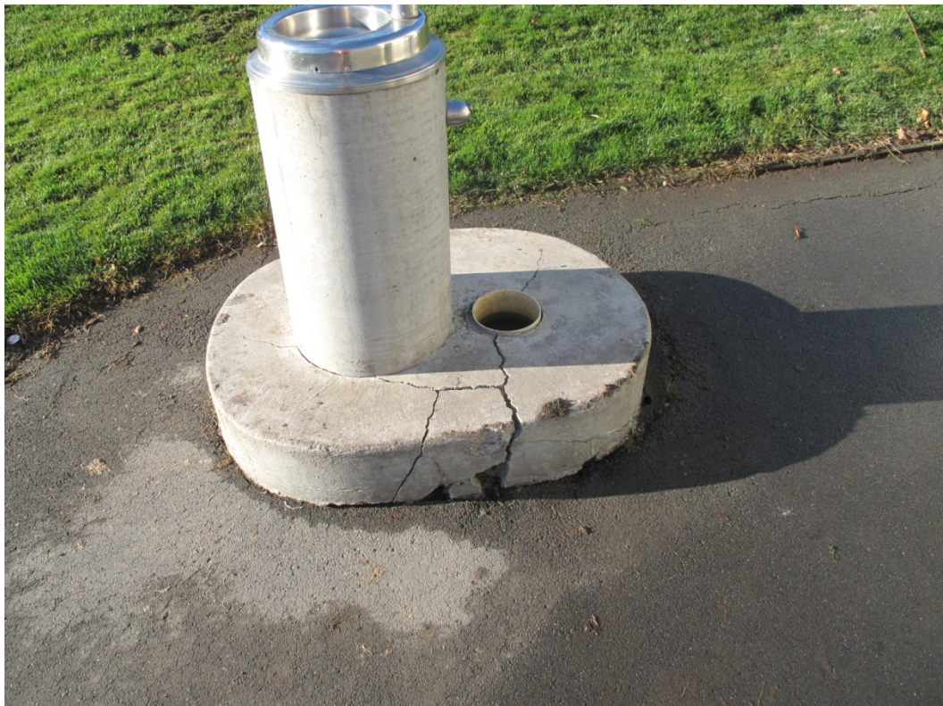
Photograph 6 Cracking and loss of concrete in base of drinking fountain.
