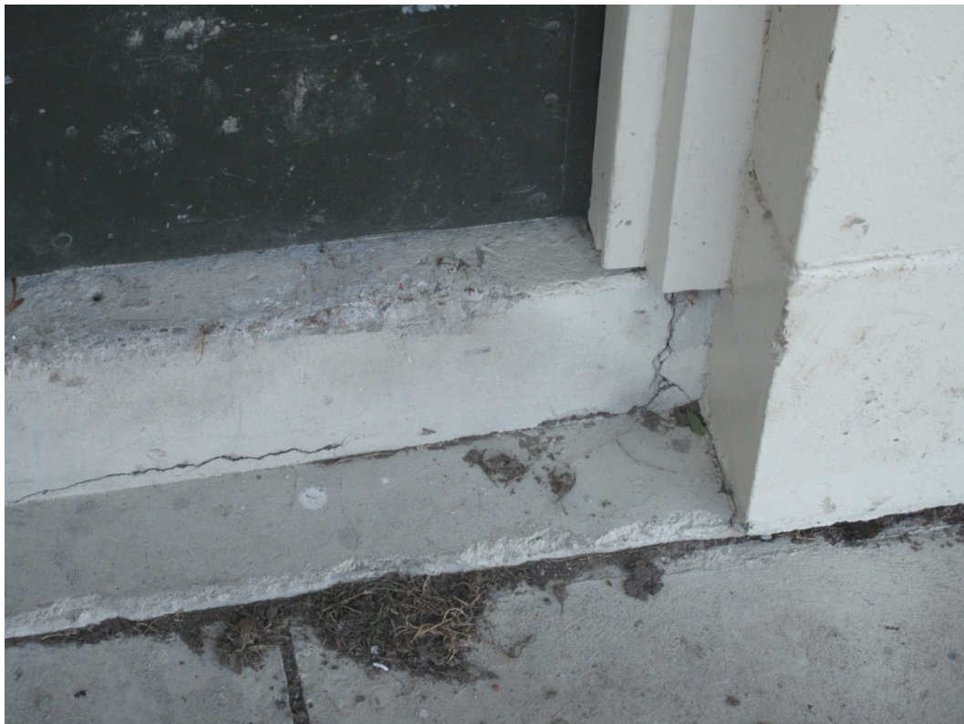
Photograph 4 Minor cracking at edges of slab on grade
