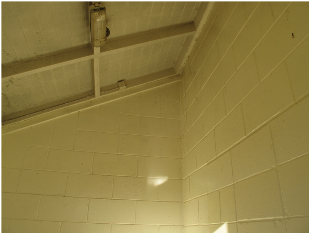
Photograph 8 Timber beam on the back wall connecting the roof to the block walls.
