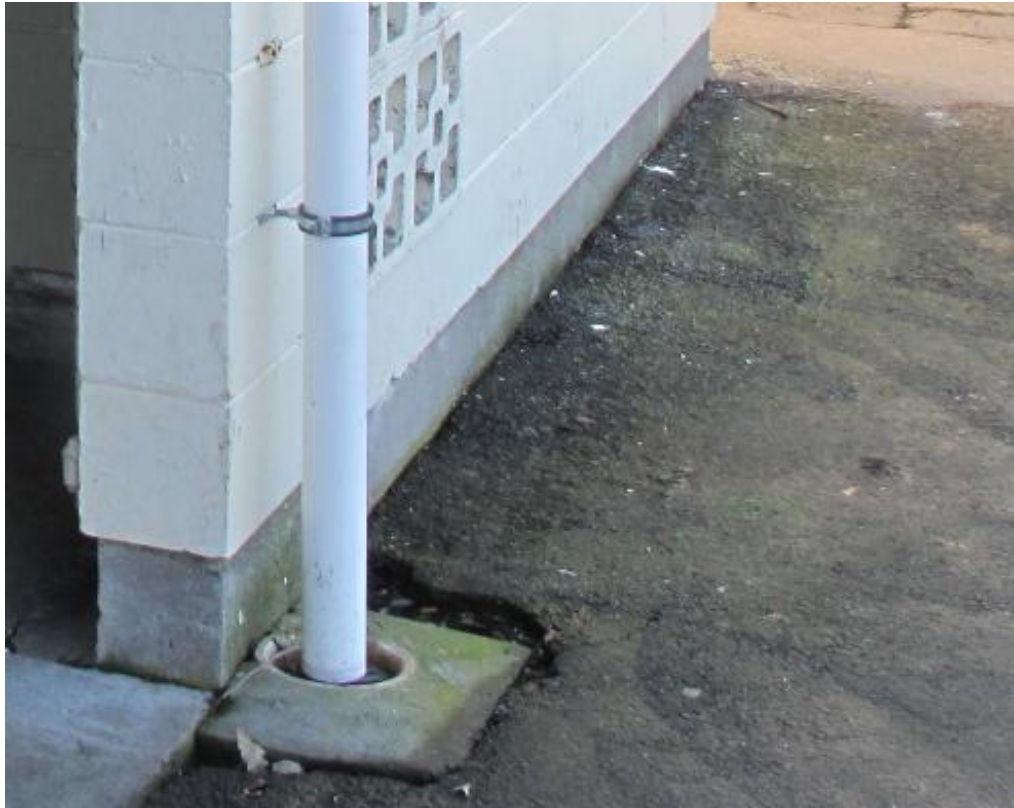
Photograph 7 Southern edge of toilet area. Note differential settlement in slab.
