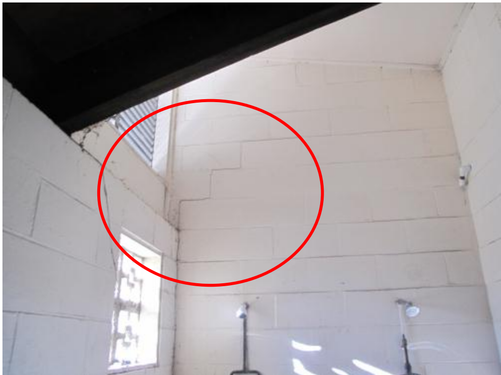
Photograph 8 Step cracks in Wall 2 due to lean in external Wall 7.
