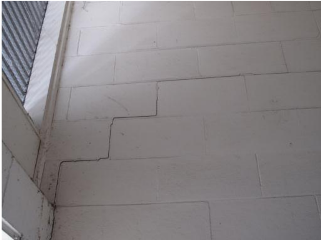
Photograph 9 Step cracking extends above the level of external wall 7.
