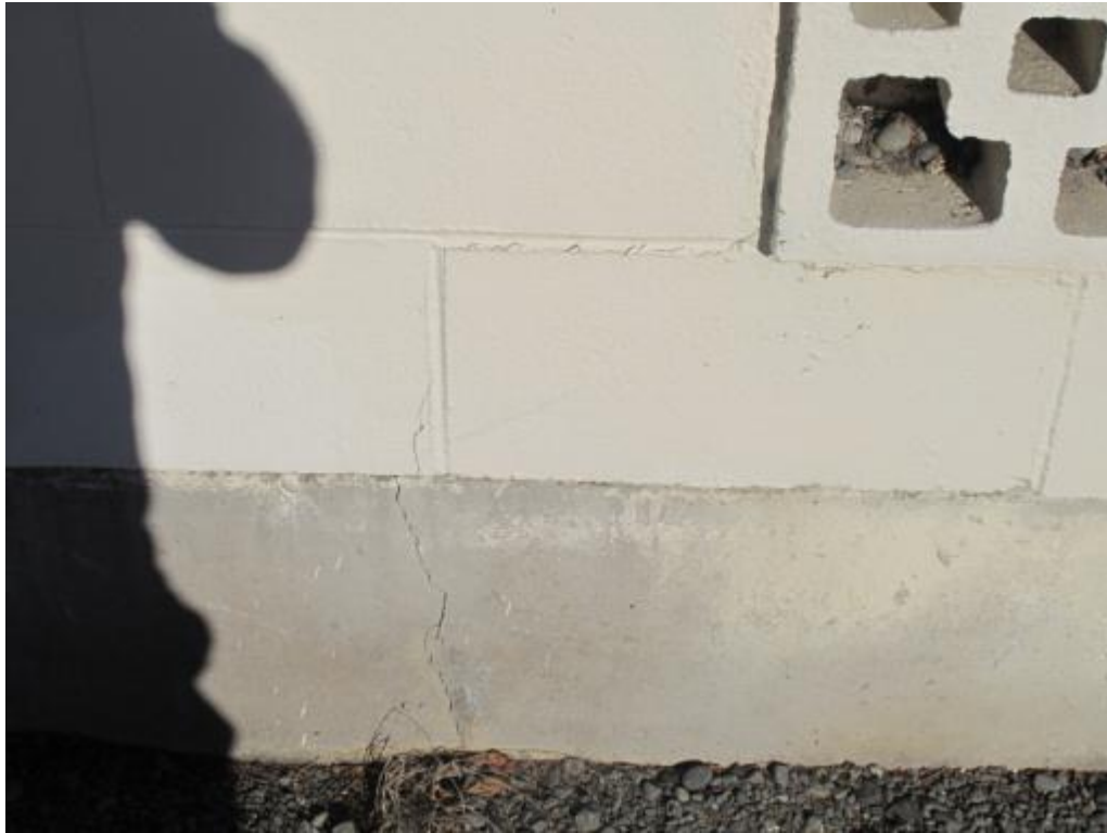
Photograph 11 Cracking in slab at base of section where Wall 2 and Wall 7 intersect.
