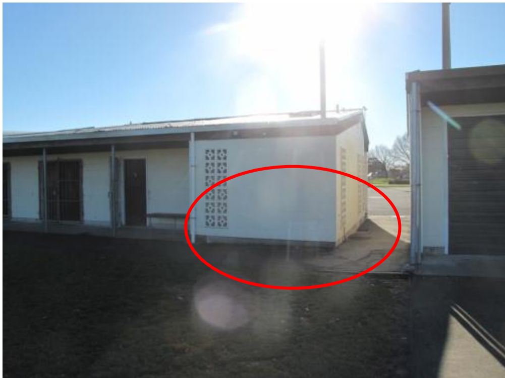
Photograph 6 Eastern end of building where settlement has occurred.
