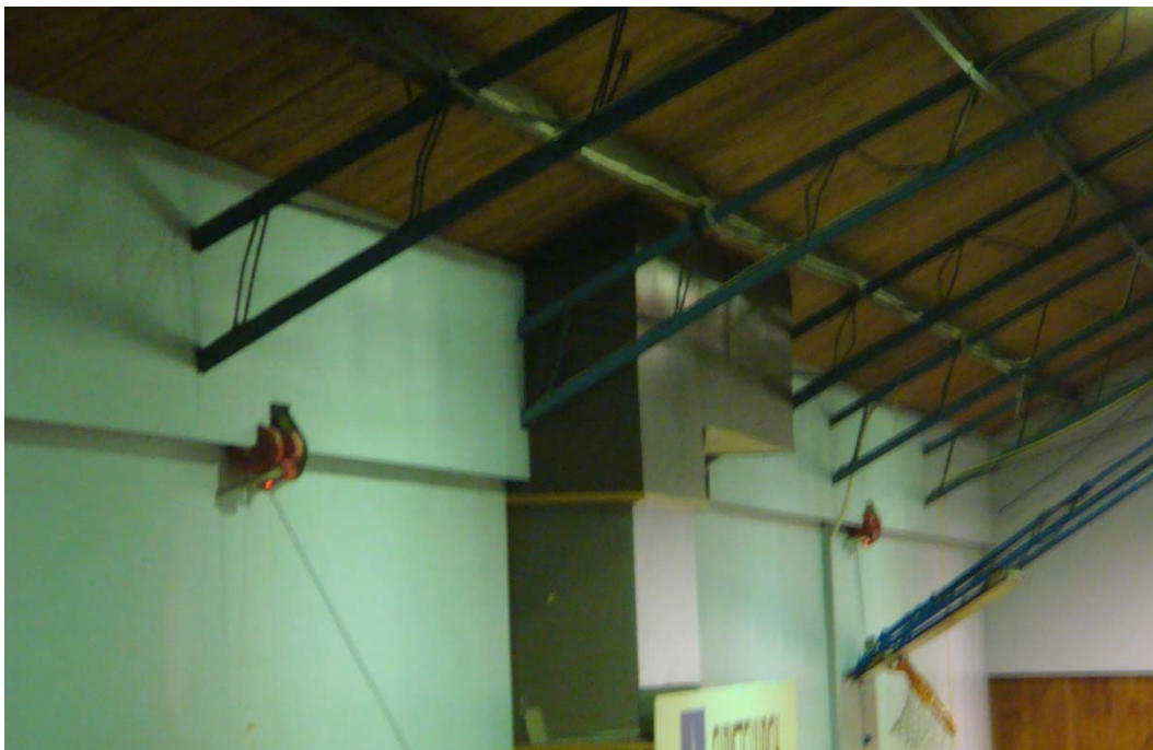
Photo 4 Buckled web members
