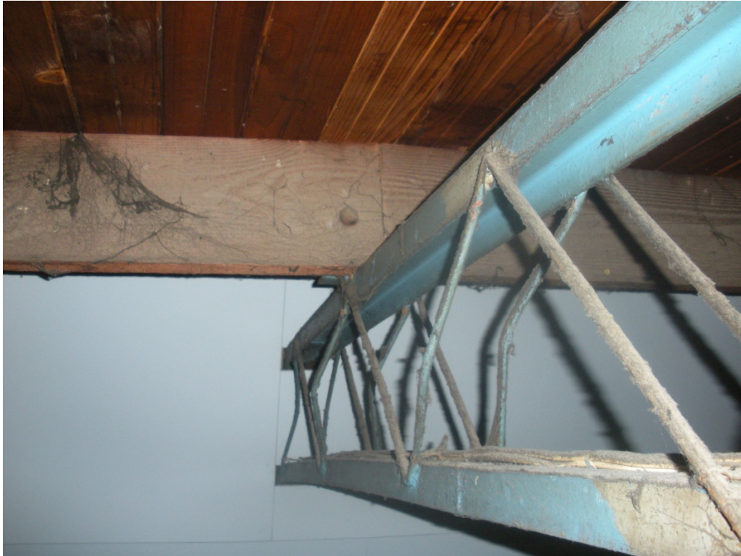
Photo 3 – Buckled web members and bent lower chord
