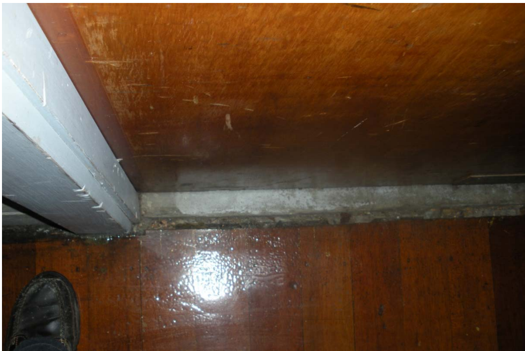
Photo 6 – Movement of South-West wall
