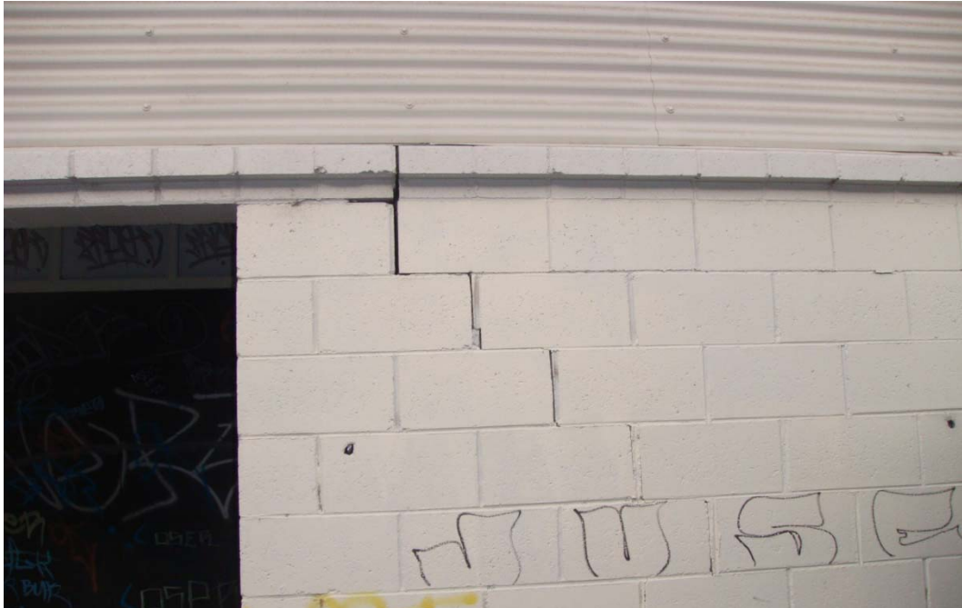
Photo 5 – Typical external wall cracking
