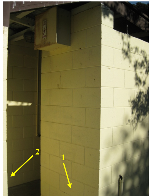
Photo 8: Hairline Cracking along Mortar Joints
