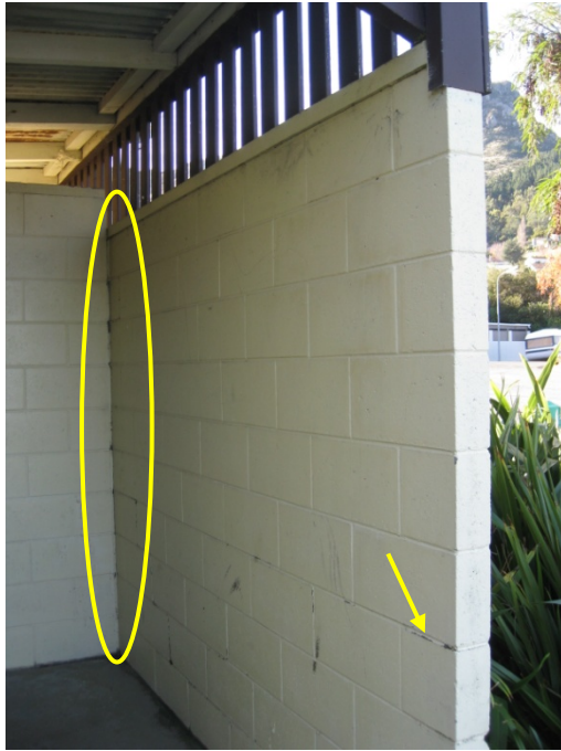
Photo 21: Hairline Cracking along Mortar Joints on East Wall of Gents
