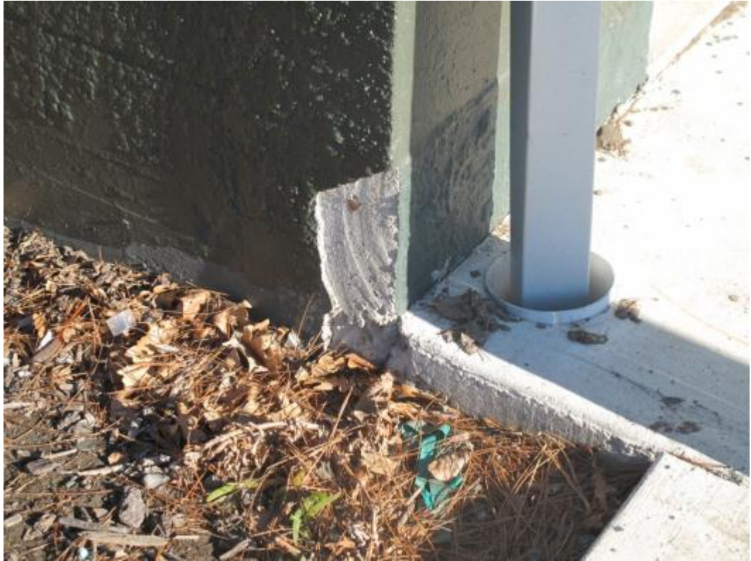
Photograph 7 Cracking of concrete slab at joint with concrete apron
