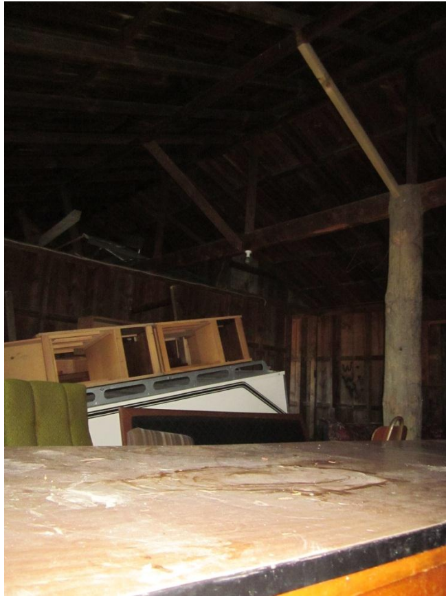
Photo showing a column, beam and struts holding up a timber roof made of timber rafters and purlins.
