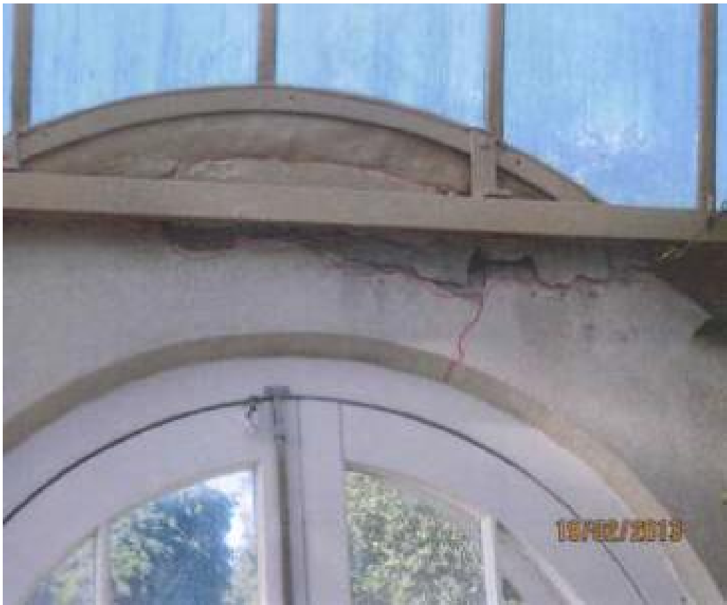
CRACK TO DOOR HEAD
