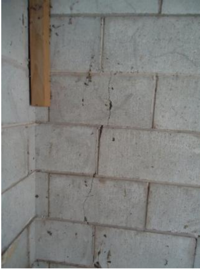
Photograph 13: Interior view of damage to north eastern wall.
