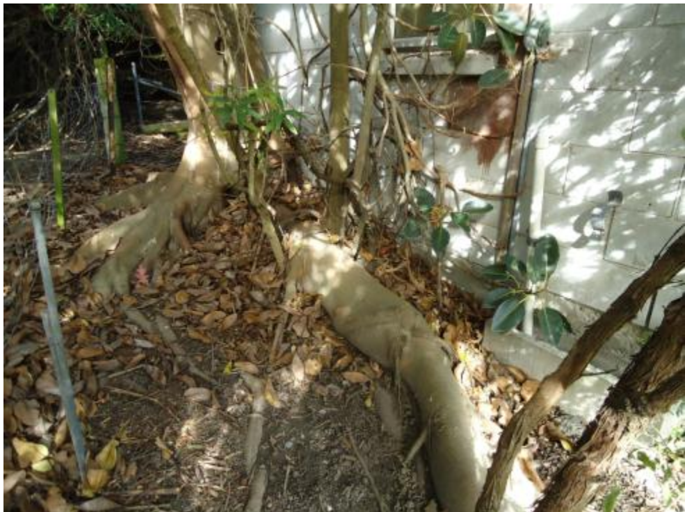
Photograph 4: Northern wall damaged by tree roots.
