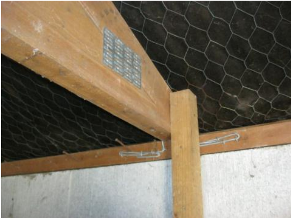
Photograph 11: Typical timber roof truss attachment to top plate on external concrete masonry walls.
