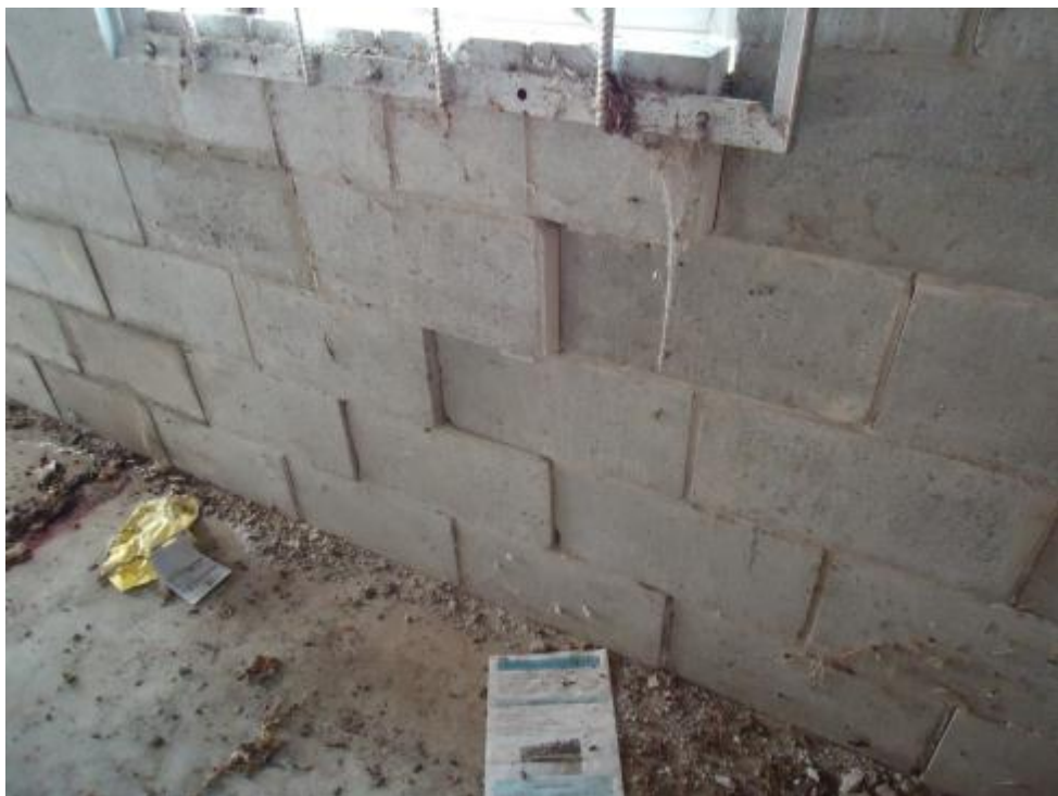
Photograph 12: Interior view of displacement to western wall by window adjacent to the north western corner of the building.
