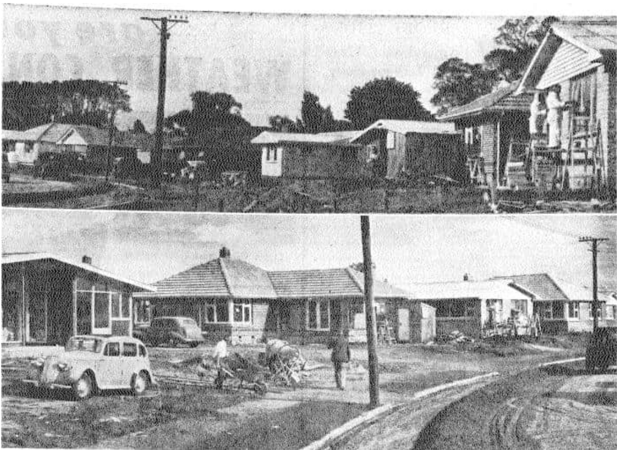
'Some of the houses which are being built in Wayside Avenue'. Press 8 March 1957, p. 7. PapersPast.
