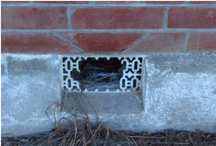
Source: B.Dougan 31/3/2015 Note the careful brick detailing with the use of English bond brick laying techniques commonly used for principal wall construction, cut and key-stoned bricks above foundation vents. From anecdotal evidence, the vents were knocked in very early after the building's construction, soon after its construction.
