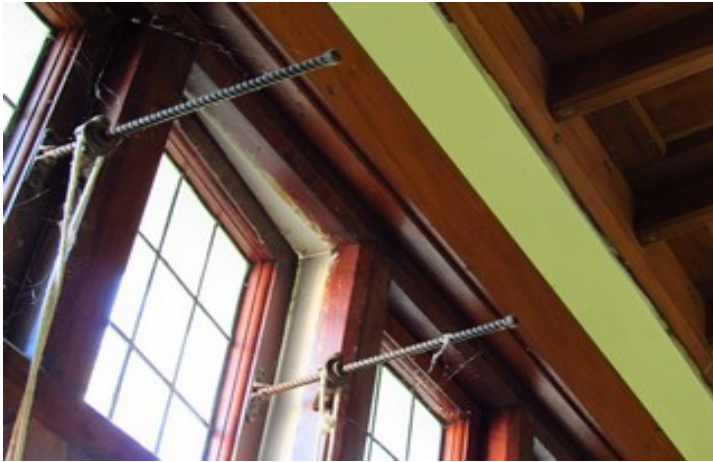
Source: B. Dougan 31/3/2015 The window catches and latches and worm gear for opening side hung toplights.
