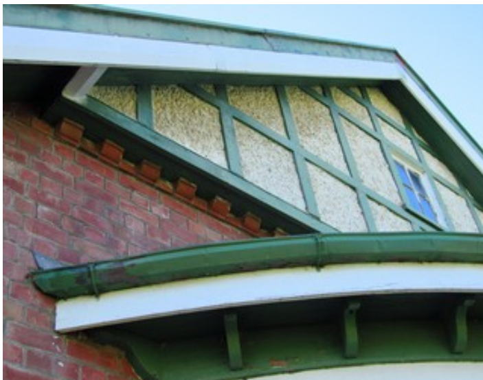
Source: B.Dougan 31/3/2015 Off the shelf brick quoins to the underside of the stippled plaster gable. The painted copper spouting is original heritage fabric
