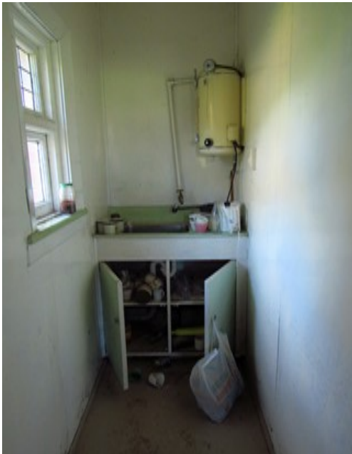
Source: B.Dougan 31/3/2015 Tearoom showing painted hardboard lining overlay to brickwork walls, crude sink bench and poorly executed plumbing. All of this is non-original fabric or no heritage value.
