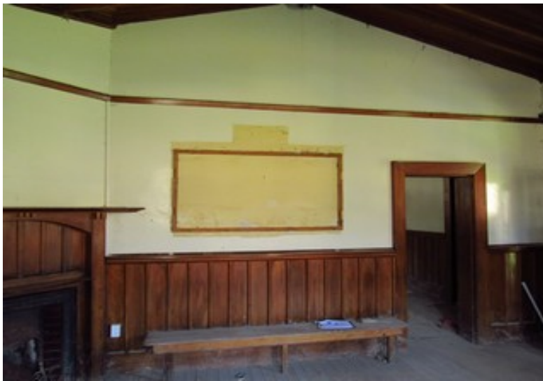
Source: B. Dougan 31/3/2015 West wall of the Reading Room. The timber frame held one of the memorial boards that were displayed in the Reading Room. The yellow ochre paint to the walls within the frame appears to be original wall colour. The Rimu panelled dado to the walls encircle the room
