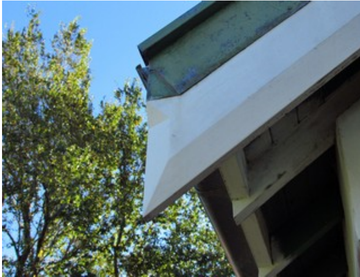
Source: B.Dougan 31/3/2015 The shaped barge boards exhibit the legacy of Arts and Crafts style craftsmanship
