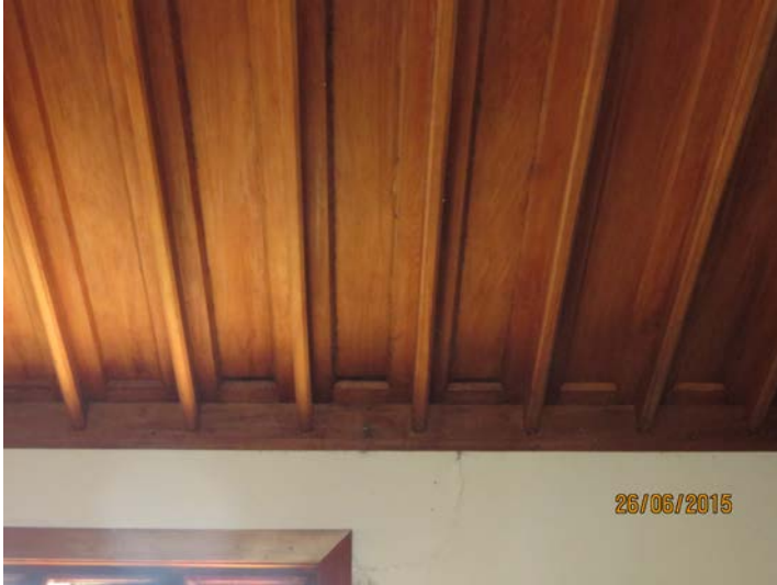
Source: T. Ussher 25/6/2015 The ceiling of the Library Room showing the raised panels creating a ventilation gap.
