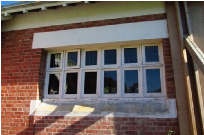
Source: B. Dougan 31/3/15 The north windows to the Library room showing weathered paint to the plastered sills. Note the side hung toplights.
