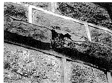
Spalling tuff string course & poor plaster repair
