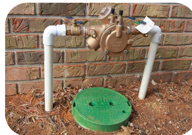
Backflow Prevention Device
