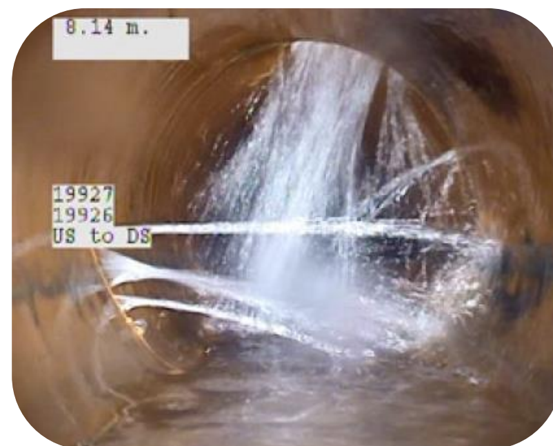
Groundwater entering through cracked pipes
