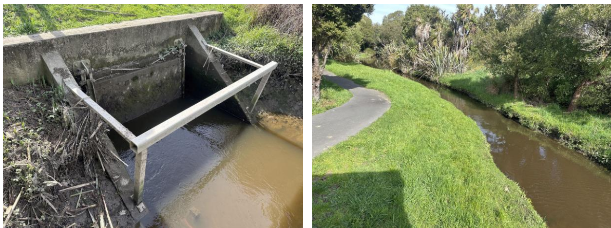
Figure 8: The Corser Stream flap gate (left) and Corser Stream, upstream of the flap gate (right).
