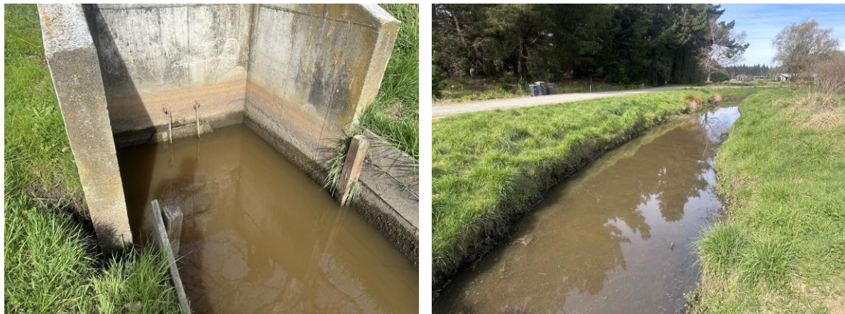
Figure 3: The Sheppards Drain flap gate (left) and Sheppards Drain upstream of the structure (right).
