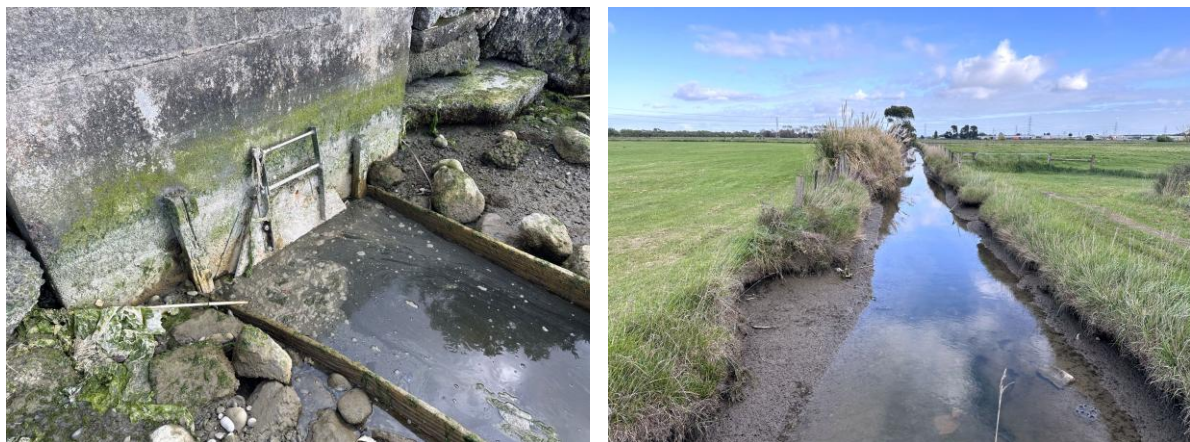
Figure 5: The flap gate outlet of Lovetts Drain (left) and upstream habitat (right), during the October 2024 visit (incoming tide).
