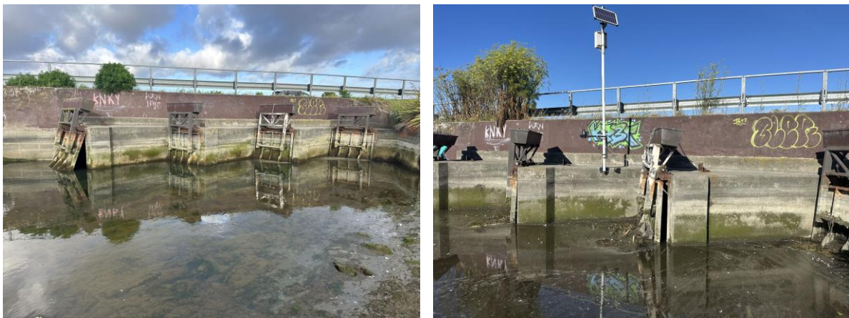
Figure 7: The tide gates in Linwood Canal (left), including the water level and gate angle sensors associated with the ongoing study (right).
