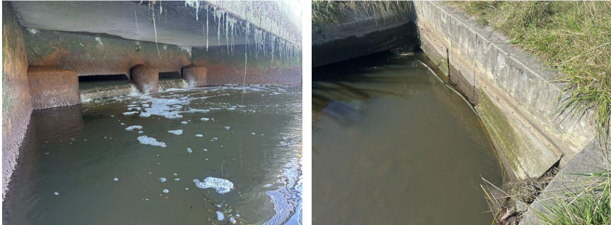
Figure 9: The Lake Kate Sheppard outlet structure, including the discharge into the Avon River (left) and the upstream flow-restricting flaps (right).
