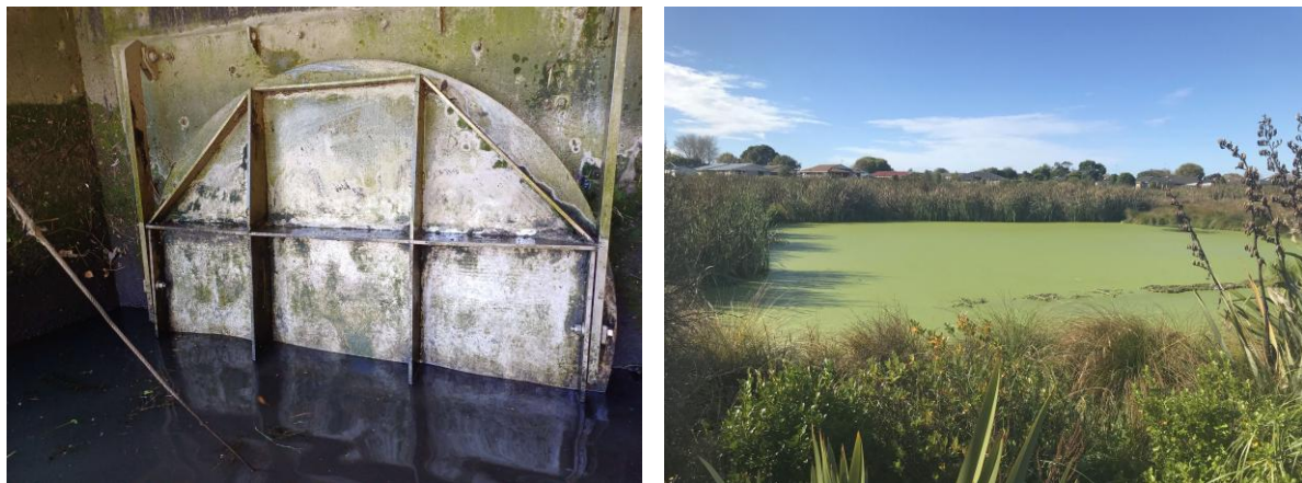
Figure 4: The Bells Creek tide gate (left; photo provided by Colin Hill, CCC) and the upstream Te Oranga Waikura stormwater wetland (right).
