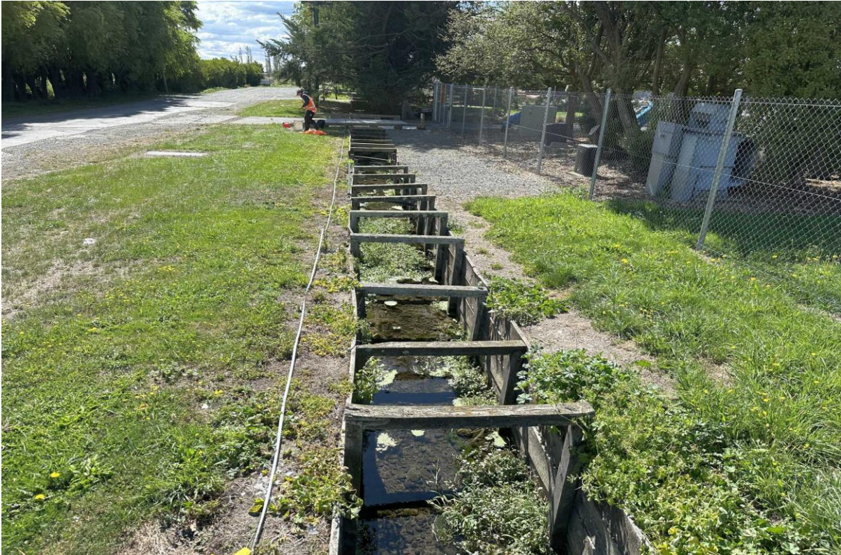
Figure 4: OTUKAI06 (Wilson's Drain at Tyrone Street). Upstream end of reach looking downstream.
