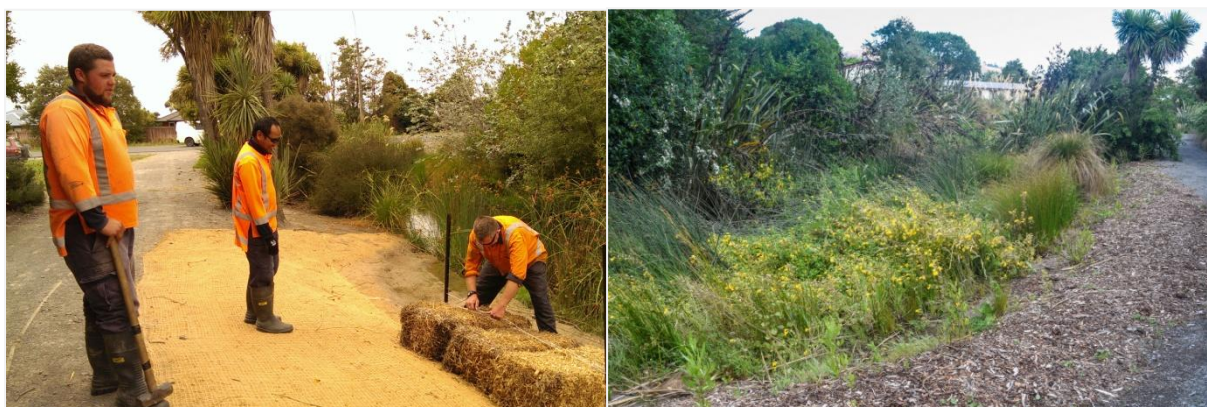
Fig. 2. (a) Bank stabilisation restoration work in 2018, which included the installation of straw bales as a mitigation measure to provide temporary spawning habitat. (b) View of the same site in 2020 showing newly established rushes, Carex and riparian herbs.
