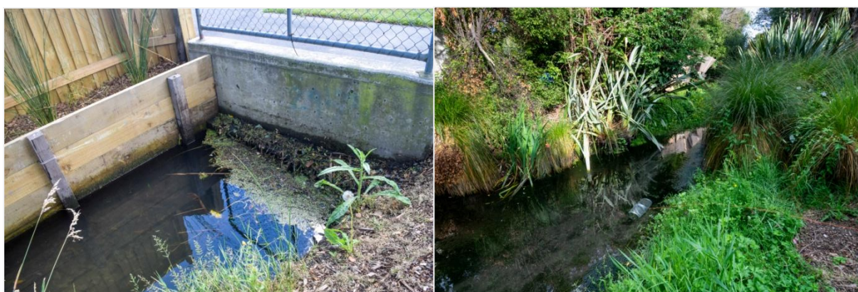
Fig. 3. (a) Alport Place box culvert showing the outlet structure which is fully submerged at typical water levels. (b) Steamwharf Stream in the reach below Alport Place at a GMT (minnow trap) sampling point.
