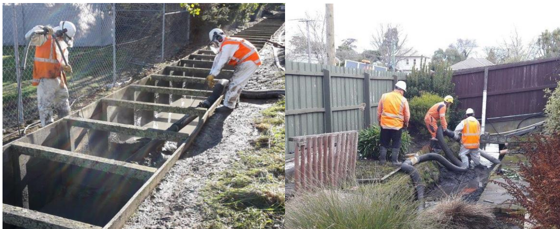
Figure 5-2: Use of water blaster and vacuum hose to remove fine deposited sediment from Jarden’s drain (left) and vacuum hose to remove sediment from St Albans Creek. Photos provided by CCC.
