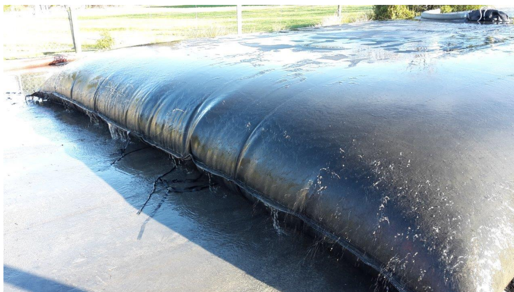
Figure 5-5: Geobags are an option to contain fine sediment mobilised during removal operations or instream works. Using baffles and filters such as hay bales to contain fine sediment mobilised during excavator works can be challenging in larger waterways. In smaller reaches pumps can filter some slurry through geobags, where the water drains from the bag leaving the sediment inside. Dried bags can then be disposed of. However, in larger waterways or remediation works this method is challenging and checking for accidental capture of sensitive taxa is difficult.
