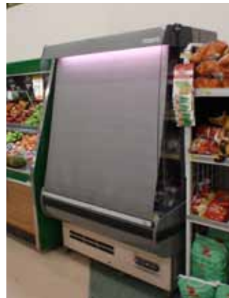
The new chiller with a night blind © Copyright
