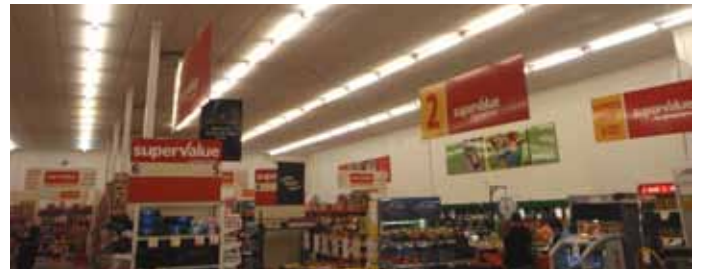
Shop floor lighting fitted with new electronic ballasts © Copyright
