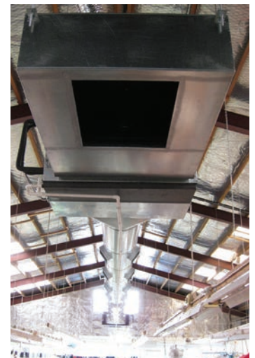
New HVAC system © Copyright
