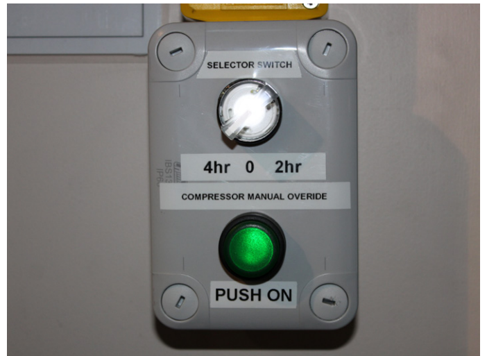
Air compressor timer switch © Copyright
