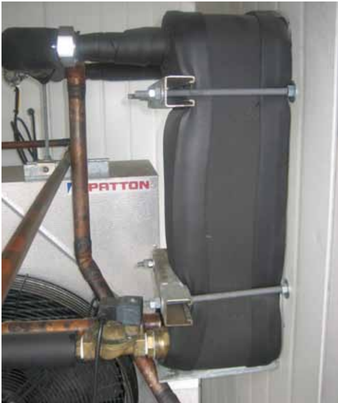
Heat exchanger where refrigerant heats cold water © Copyright
