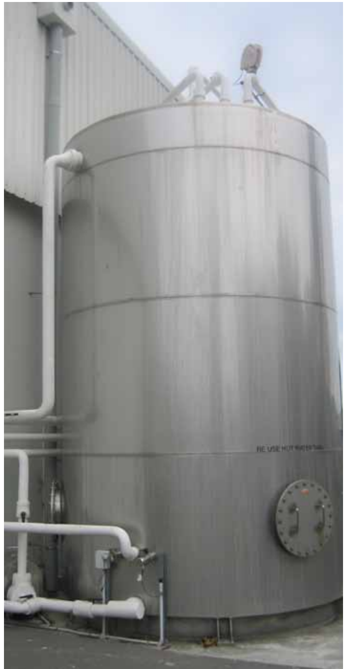
Insulated tank to store the pre-heated water © Copyright
