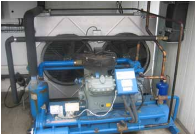
Refrigeration compressor with heat exchanger © Copyright
