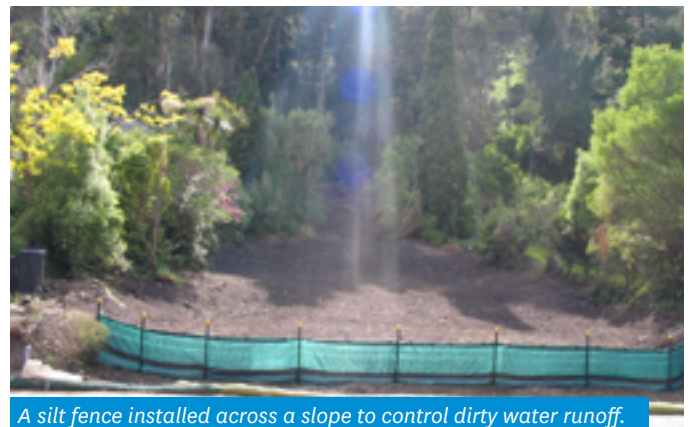
A silt fence installed across a slope to control dirty water runoff.
