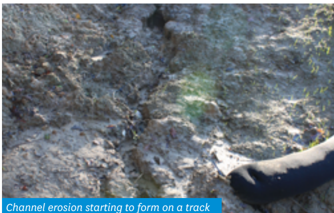
Rilling on exposed Port Hills soil
