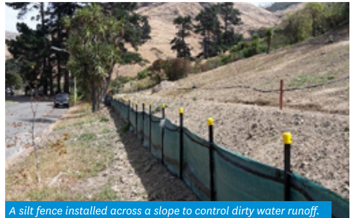
Compost silt socks with returns installed, to catch sediment eroding from the surfaces above
