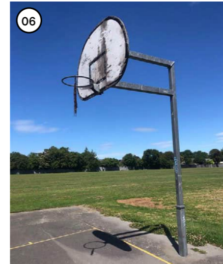
Half court surface sits within the bounds of the new court and may be refurbished. The existing hoop and back board are in poor condition. These may be re-purposed for another use.
