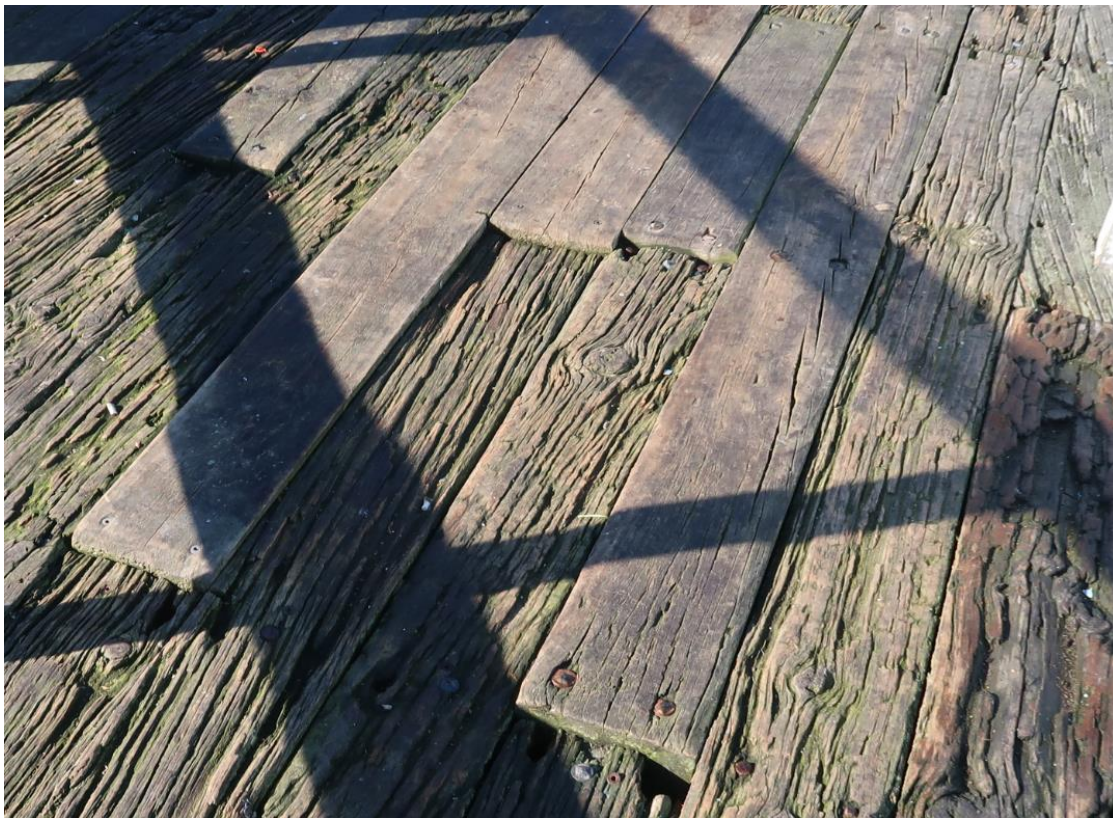
Figure 3: Mixture of old and new decking timber, with 15-20mm difference in height
