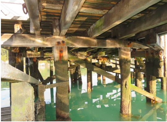
Source: T Ussher June 2020 Typical construction with piles, bracing, wharf beams and decking.
