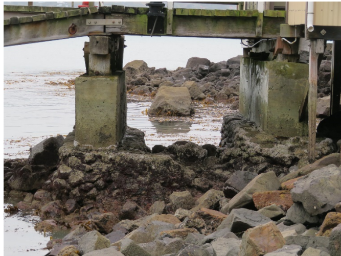
Source: T Ussher June 2020 The two lines of piles in the inter-tidal zone with the stone foundation walls and later concrete pile encasement and walls.
