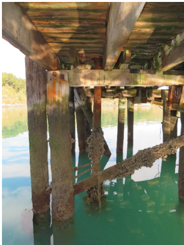
Source: T Ussher June 2020 The armature of the crane swivel below the wharf is restrained by cargo strops.
