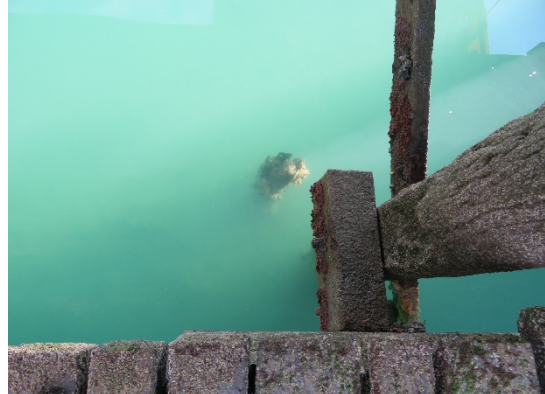
Source: T Ussher June 2020 The remains of a pile seen below the low tide water line.
