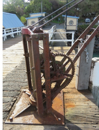
Source: T Ussher June 2020 The crane crank and winch mechanism.
