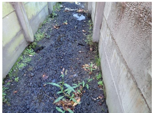
Figure 7. Damp gravel in Lydia Street Drain.
