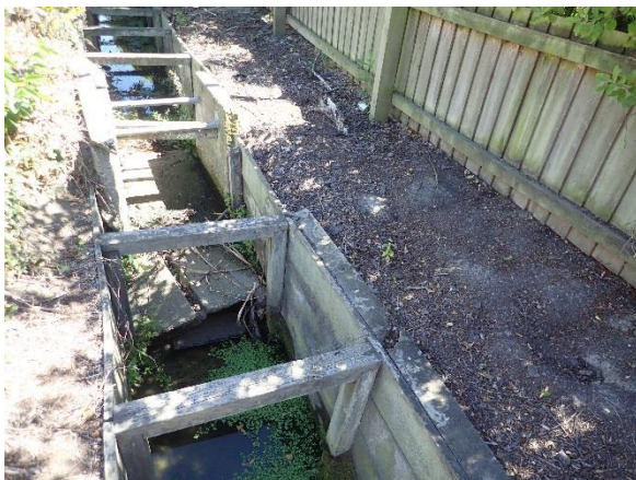
Figure 10. Concrete debris damming water in Lydia Street Drain.
