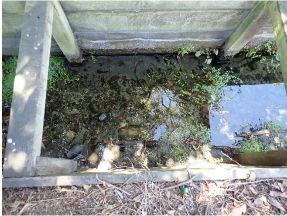
Figure 8. Embedded hard substrate in Lydia Street Drain.
