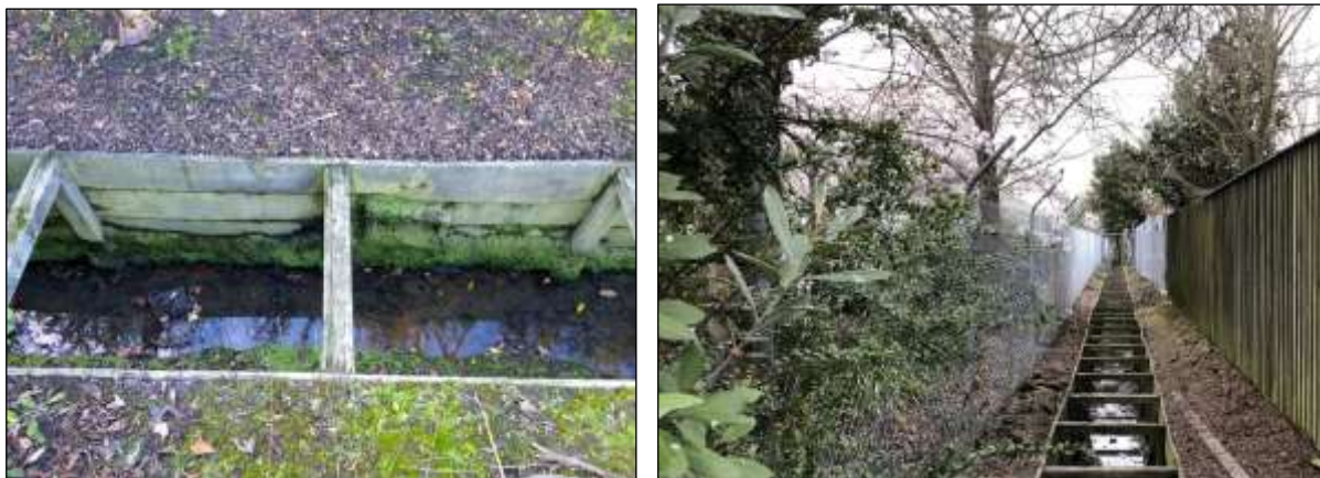
Figures 11 and 12. Lydia Street Box Drain along north boundary of the site.
