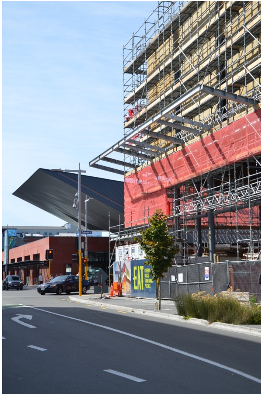
Figure 27: A view, from Lichfield Street to the west of Colombo Street, of the Entx Building's steel veranda framing and the Bus Interchange's dramatically large scale entrance canopy.
