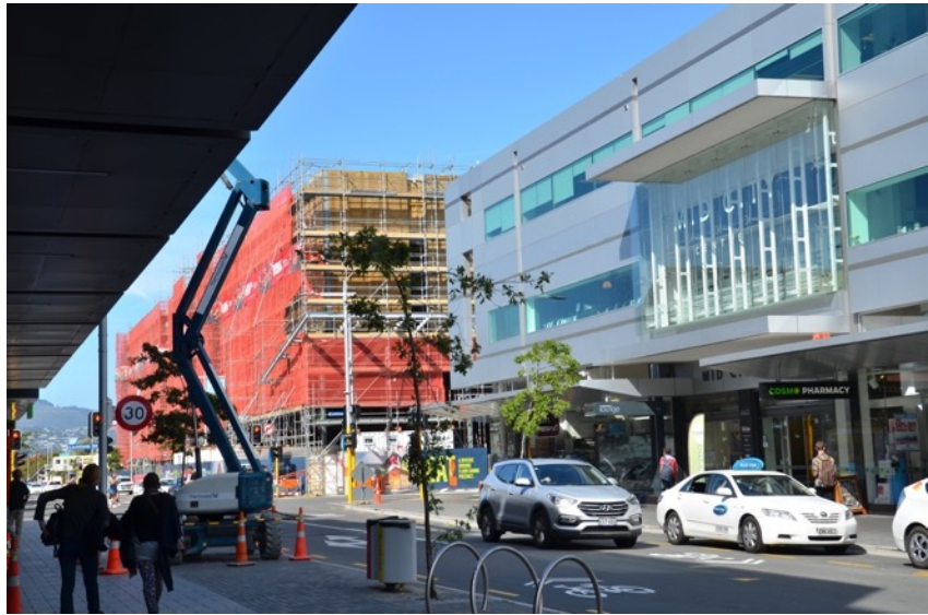
Figure 6: The renovated large, three storey Ballantynes Building , viewed from the east side Colombo Street to the north of the EntX building. Ballantynes occupies nearly half of the city block bounded by Lichfield Street, Colombo Street, and Cashel Street.
