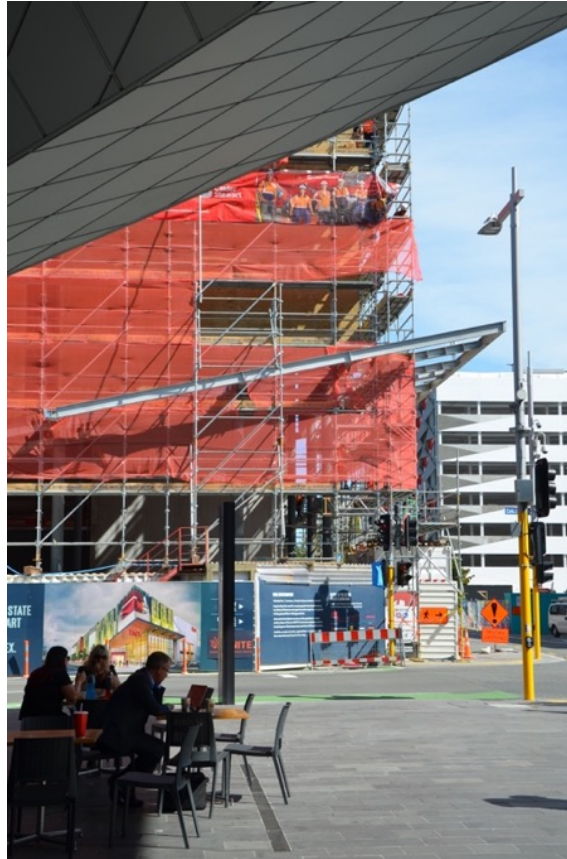
Figure 30: A view of that part of the EntX building to which the screen will be fixed (on the corner above the sloping veranda canopy), when exiting the Bus Interchange.
