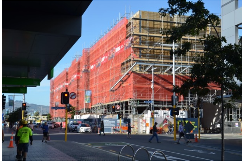
Figure 4: The EntX building, currently under construction on the corner of Colombo and Lichfield Streets, viewed from Colombo Street looking south.
