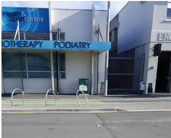
Photograph 1: Damaged Cycle Stand
