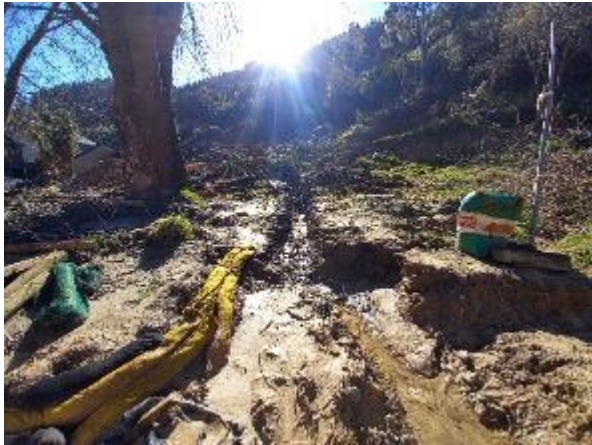
Figure 7: View of the drain dug by the customer which connects to the base of Gully B
