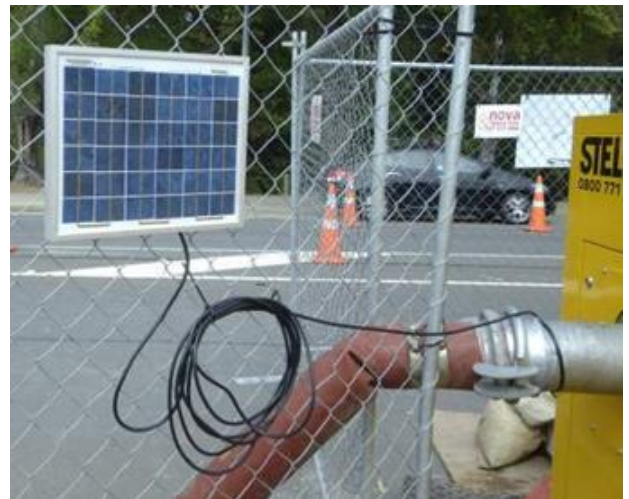
Figure 21: Solar Panel for Float Alarm
