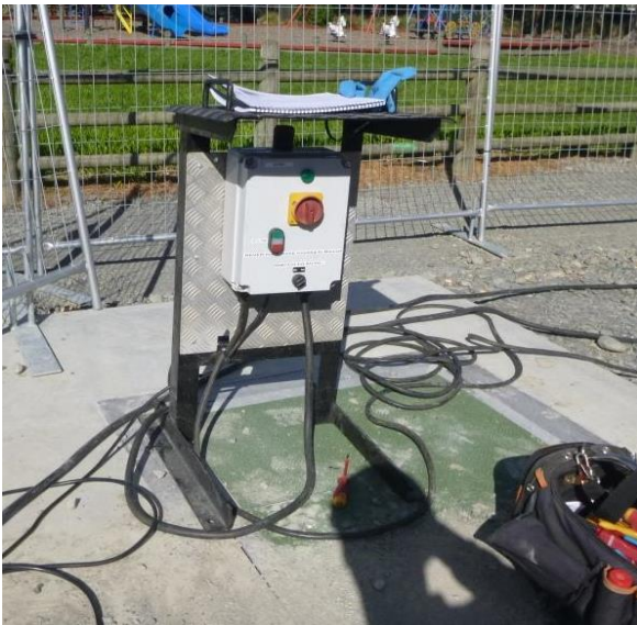
Figure 6: Electric Pump Builders Box
