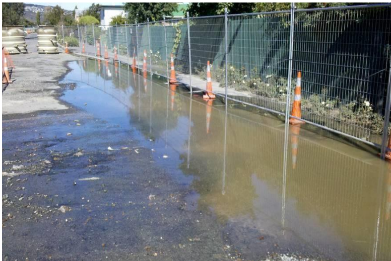
Picture 1: Wastewater ponded on street following an overflow.
