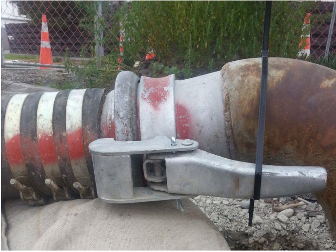
Figure 8: Layflat Pipe: Couplings secured
