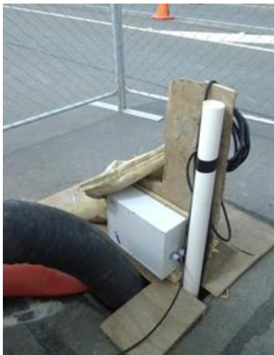
Figure 20: Float Alarm in Suction Manhole
