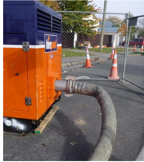
Figure 9: Layflat Pipe: Kinks can obstruct flow
