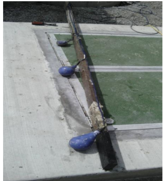
Figure 7: Electric Pump: Two Level Flow Switch
