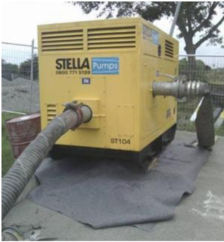
Figure 31: Spill Mitigation: X TEX Fabric under pump
