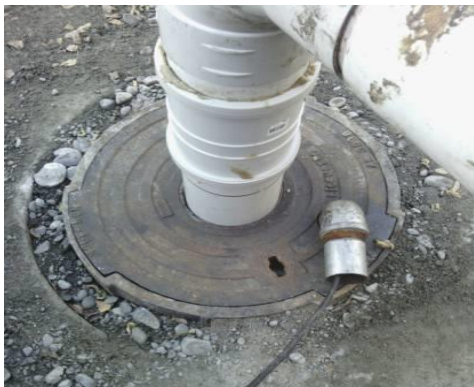
Figure 35: Manhole lid with PVC inlet
