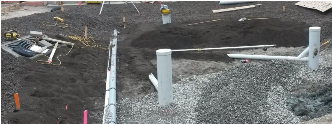
Figure 33 Install appropriate under drainage system (example in photo will have trees installed).
