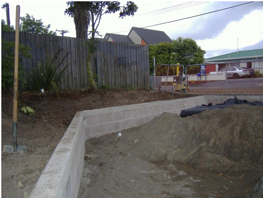
Figure 31 Construct edge walls as specified. The soil below rain garden should be loosened with teeth on excavation bucket to 300mm below surface.
