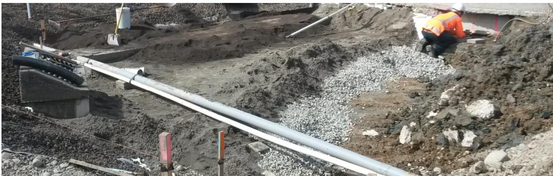
Figure 34 Place drainage layers and rain garden media from a low level and spread manually
