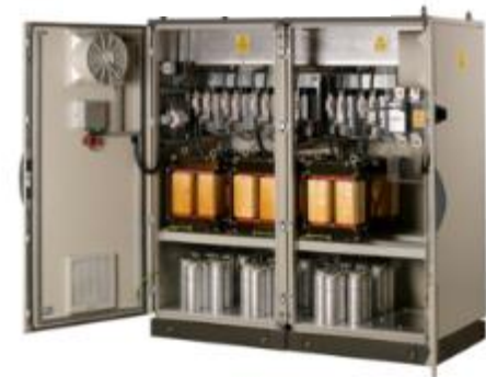
Harmonic Filter Cabinet
