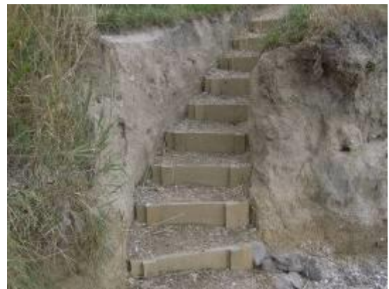
Inground stairs with no stringers.
