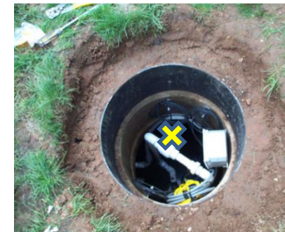
Centre of Pump X Y and Z (on pump)
