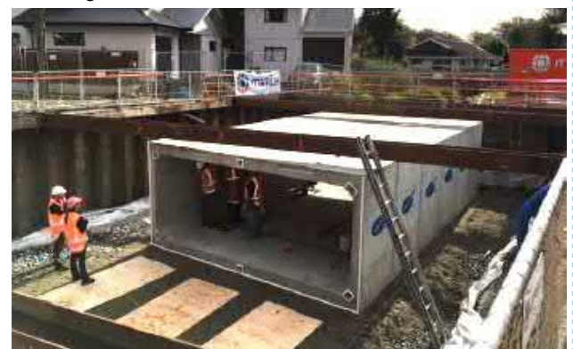
Image 1. A sheet piled trench with installed culvert, showing the width of the work site .
