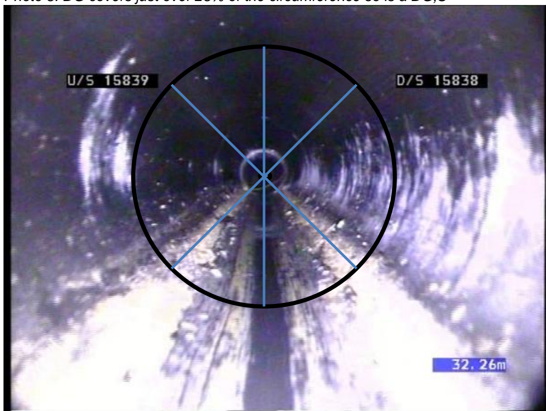
Photo 5: DG covers just over 25% of the circumference so is a DG,S
